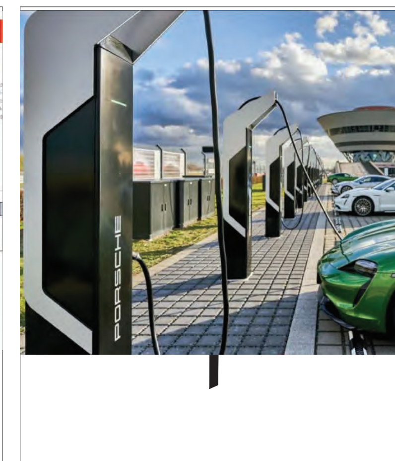
J CHARGING STATION (AC) 2 Public Accessible located on Haynes Street
